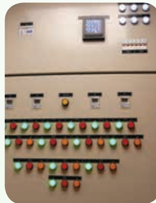
Centralised air-conditioning monitoring panel.
