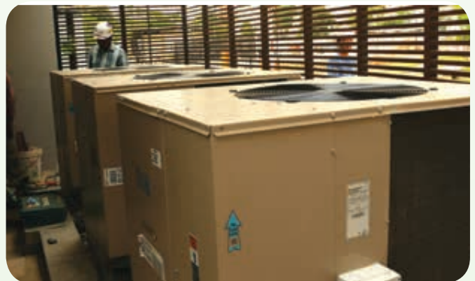
Lennox TSA 090 and 072 air-conditioning system with an average COP of 3.35.
