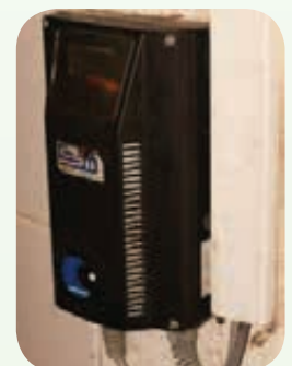
The CO 2 detector to monitor the CO 2 levels in the area where carbonated drinks are stored.
