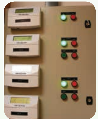
Individual air-conditioning control panels for temperature and sensor monitoring.
