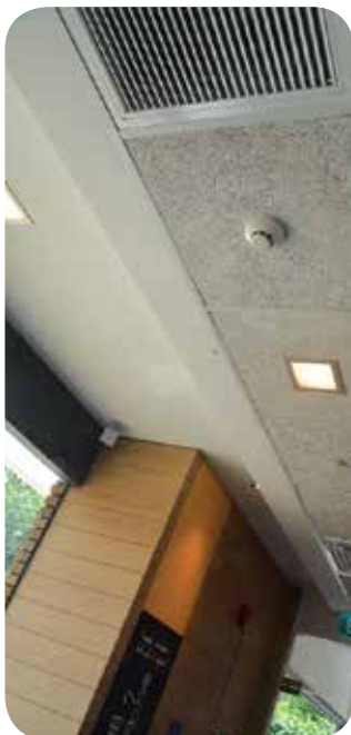
Recycled ceiling boards are used throughout the restaurant. This is a sustainable solution for improving acoustics.
