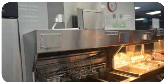
The Halton hood technology is extensively deployed in the kitchen. The canopy hood system is able to save approximately 21,120 kWh in terms of cooling load by preventing excess cooking heat from dominating the kitchen environment.
