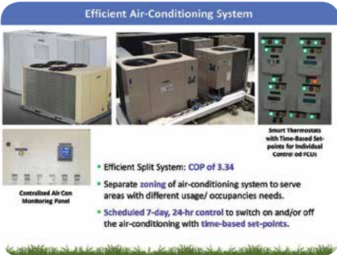
An efficient, split air-conditioning system achieves a COP of 3.34, with separate zoning to serve areas with different usage / occupancy needs. The system is scheduled for 7-day, 24-hr operation, with control of the air-conditioning achieved with time-based set-points.
